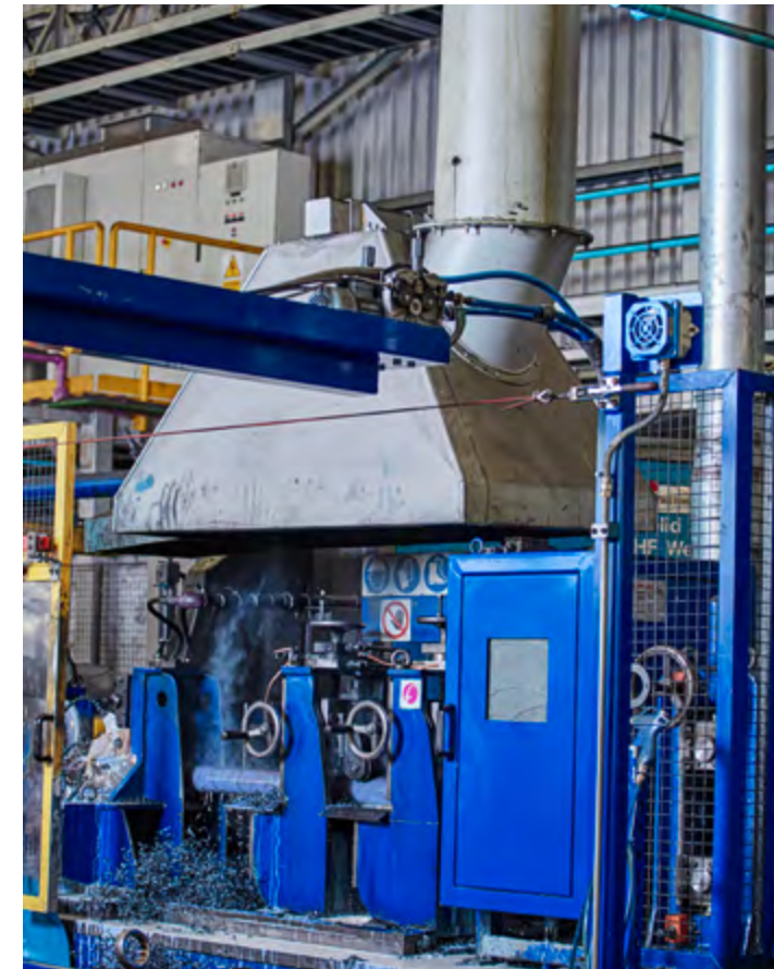
Fume extractor hood, its function is to capture the fumes, product of the welding pipe plant, extract and purify them thus mitigating the environmental impact.
